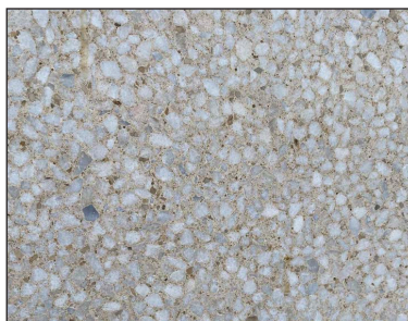
Fig. 16. Polished cement cladding at Locality 15.
