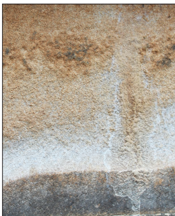
Fig. 2. Weathered Gilmorehill Sandstone at Locality 1.
